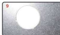
DRILLING TAP HOLE Invert the Sink, Use the marking to Drill the Hole with Wood Cutting Bit
